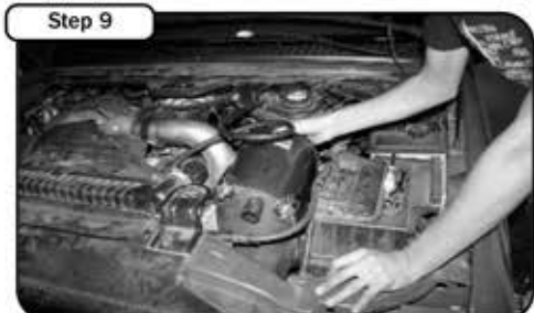
Position the inlet side of the air box assembly into the engine bay.
