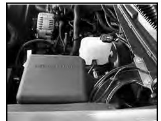
Electric Center Box Underneath Hood
