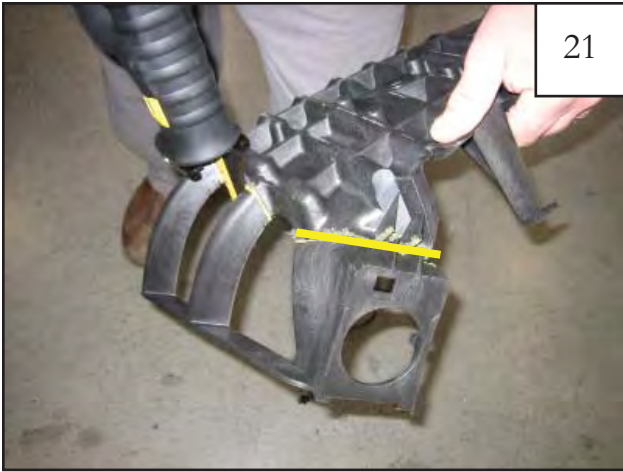
Using a hacksaw or saws all, carefully cut along lines made in Steps 19 and 20 to remove from portion of factory inner structure. Retain rearward piece.
